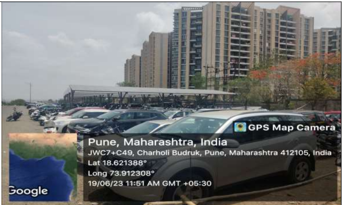
Solar Plant with Parking
