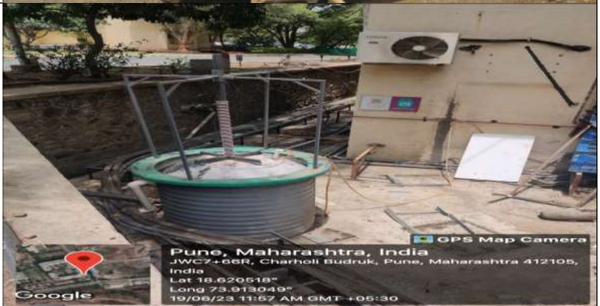
Bio gas plant
