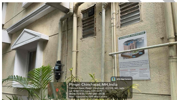
Fig1: Rainwater Harvesting Pipe with sand filter
