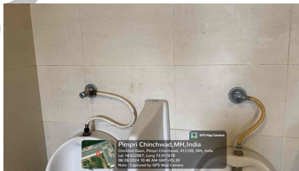
Fig2: Low water fixtures in toilets
