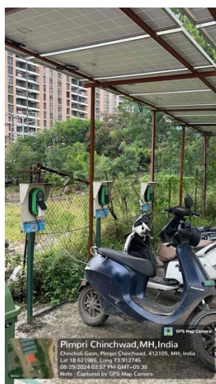
Fig1: electric vehicle charging station
