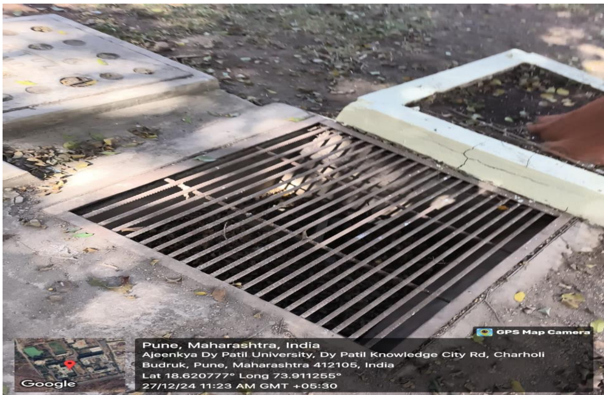
Road Cross Drainage Work which was connected to the chambers located in the campus
