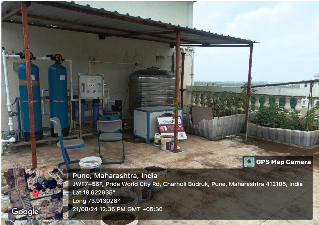
Overhead Water Tank Fitted with R.O. System
