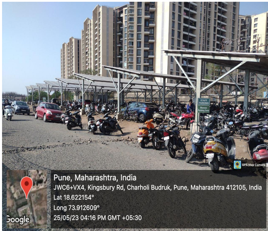
Solar Panel located at Parking Area
