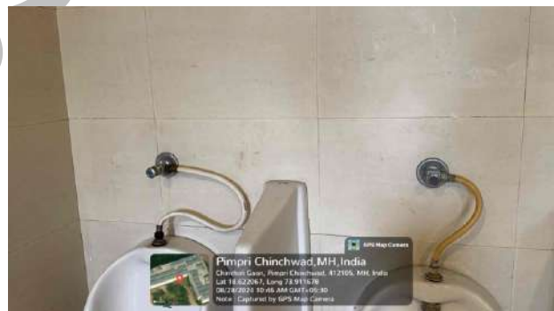
Fig2: Low water fixtures in toilets
