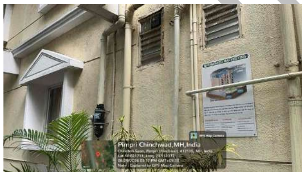
Fig1: Rainwater Harvesting Pipe with sand filter
