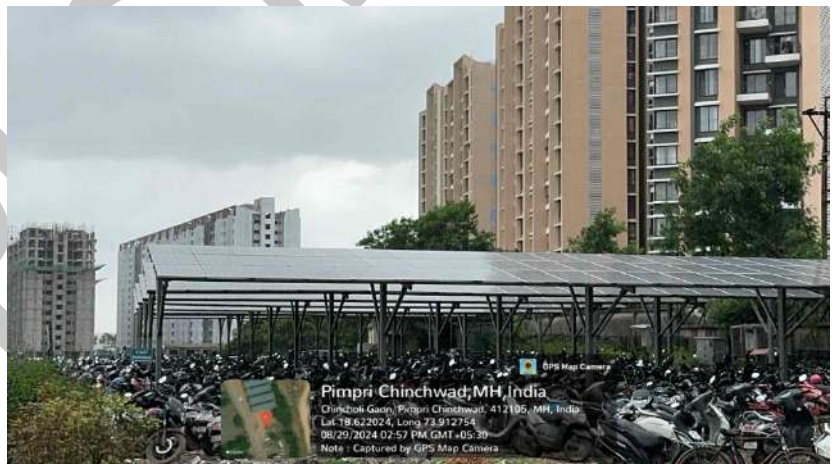
Fig2: Solar panels in parking
