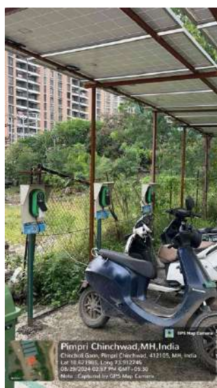
Fig1: electric vehicle charging station
