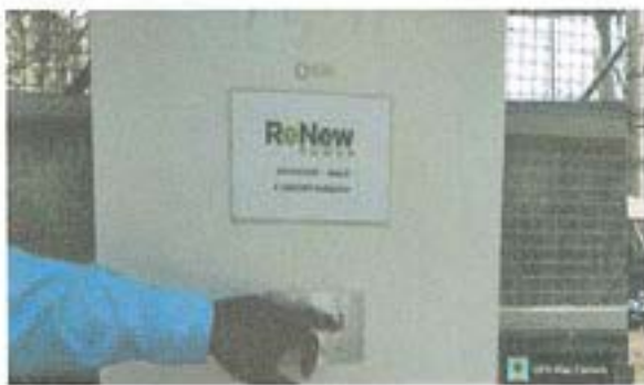
DC to AC Conversion- Inverter (60 KW)
